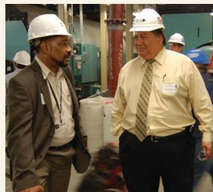
Ronald Berry (left), TWTC, and Jim Weinold, Bear Construction, tour the new central utility plant at the 2nd Quarterly meeting. (Above) Palos Community Hospital's new plant, now online, connects to the existing hospital building through an underground tunnel.
