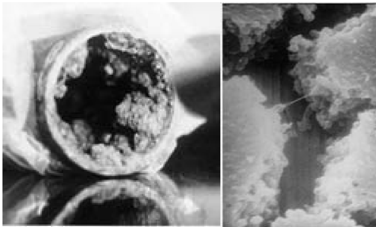
Figure 2. Left: Tubercle formation in a carbon steel fire protection pipe. Iron oxidizing bacteria were found in association with the tubercles. Right: Bacterial biofilm associated with stainless steel tube. Scanning electron micrograph magnification at 5,000X (Mittelman, 2001).
